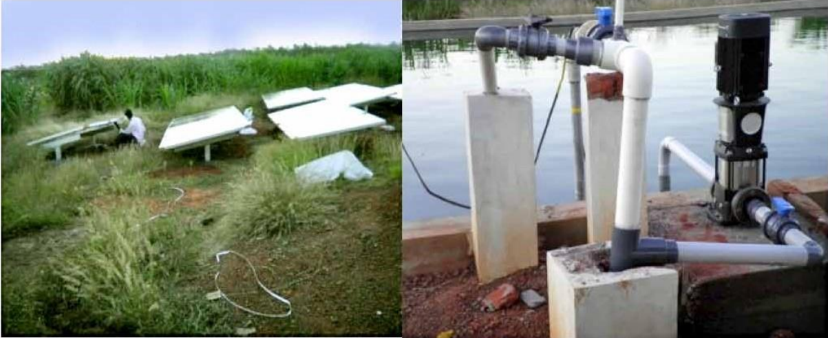
Sivaganga, TN (Irrigation 180,000 LPD @ 30 M, 4 KW)
