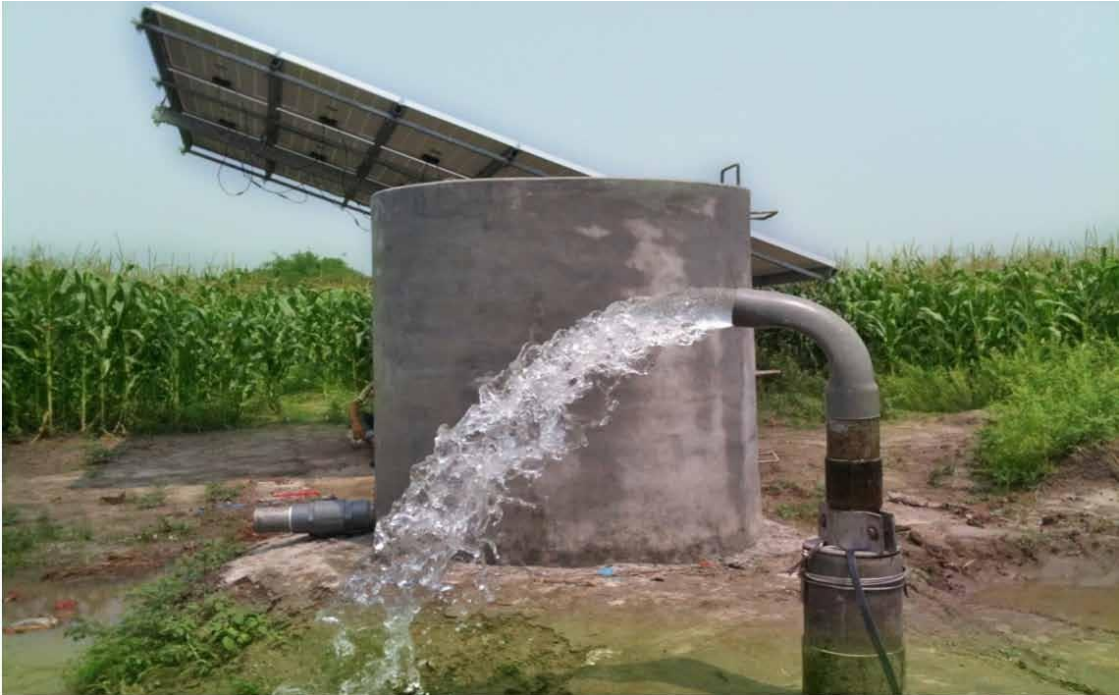
Bangladesh : Irrigation Project. SP60-3, 5.5KW, 300,000 LPD @ 20m
